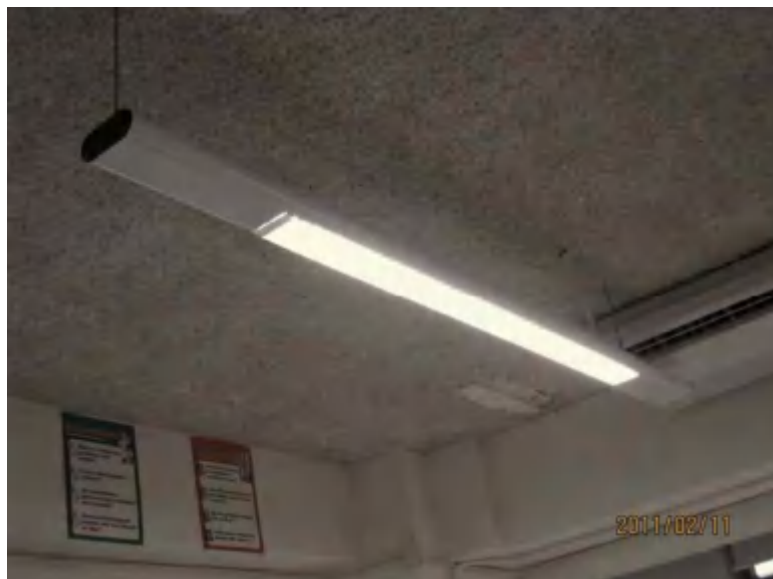
T8 Lighting before retrofit
